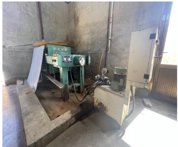
污水污泥压滤
